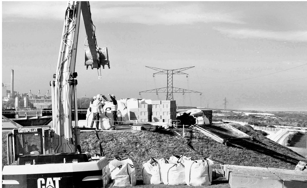
Facility being built for storage of spent fuel in La Manche, France. With the planned ramp-up in nuclear power generation, India will need to have specialised waste processing facilities too. — AFP
